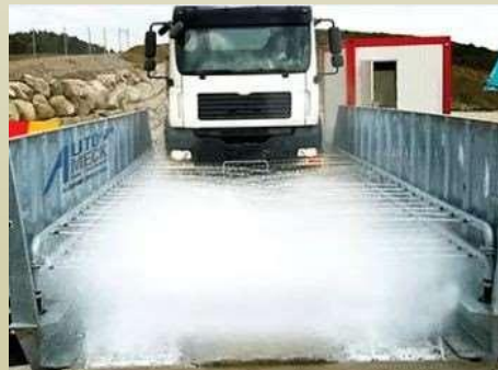
Wheel Wash System
